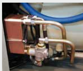
Recovered thermal energy \geq 80
